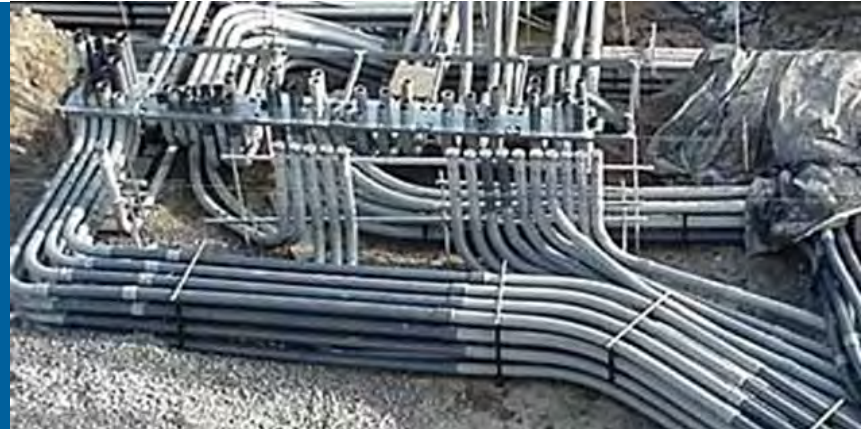
Complicated power distribution infrastructure (AC vs DC)
